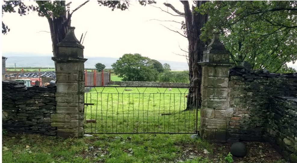
Figure 8 One of the pairs of grade II listed gate piers, to the east of the castle ruins
